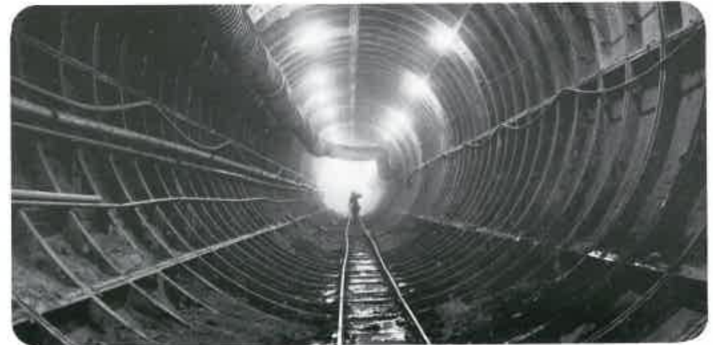
After the tunnels are bored a lining is fitted—in this case cast-iron segments.
