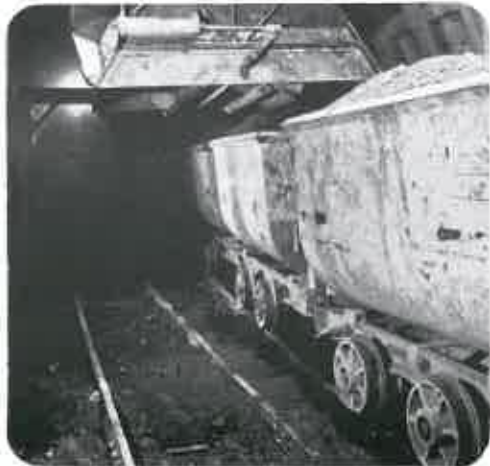
Temporary track is laid in the tunnels for removing skip loads of soil.
