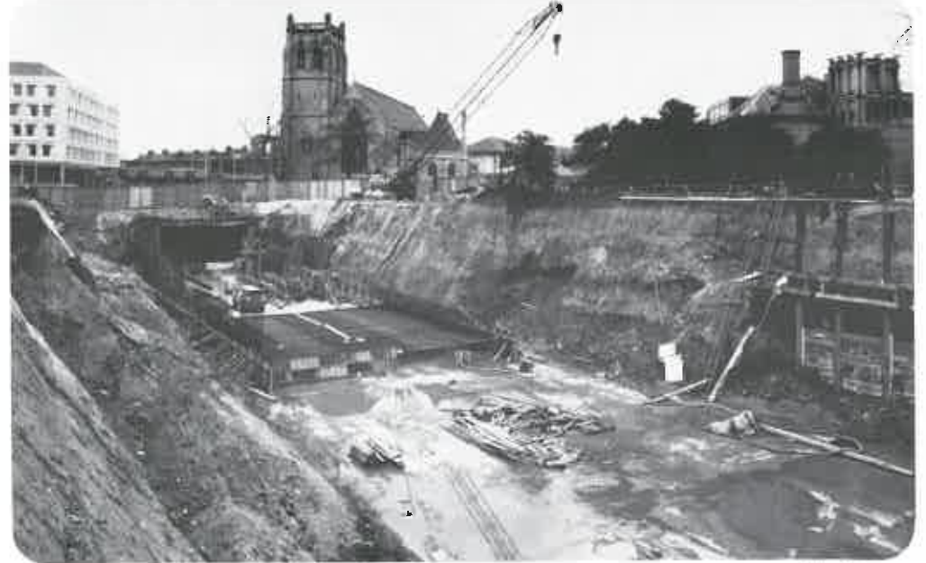
Some of the first building work on Metro was construction of tunnels under the motorway—like this one at Jesmond.
